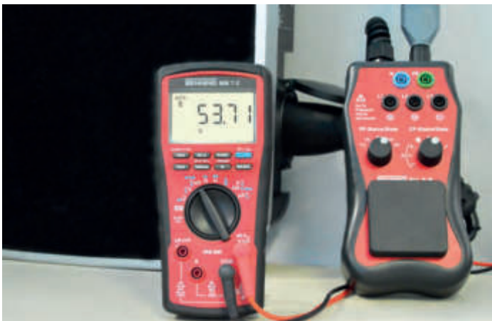
duty cycle measurement of the CP control signal of a wall box
