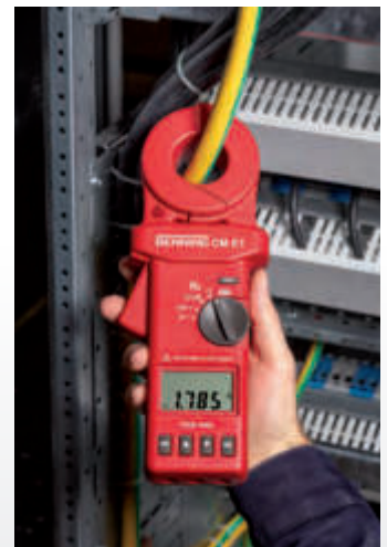
Measuring the system earthing connection of an industrial power distribution system
